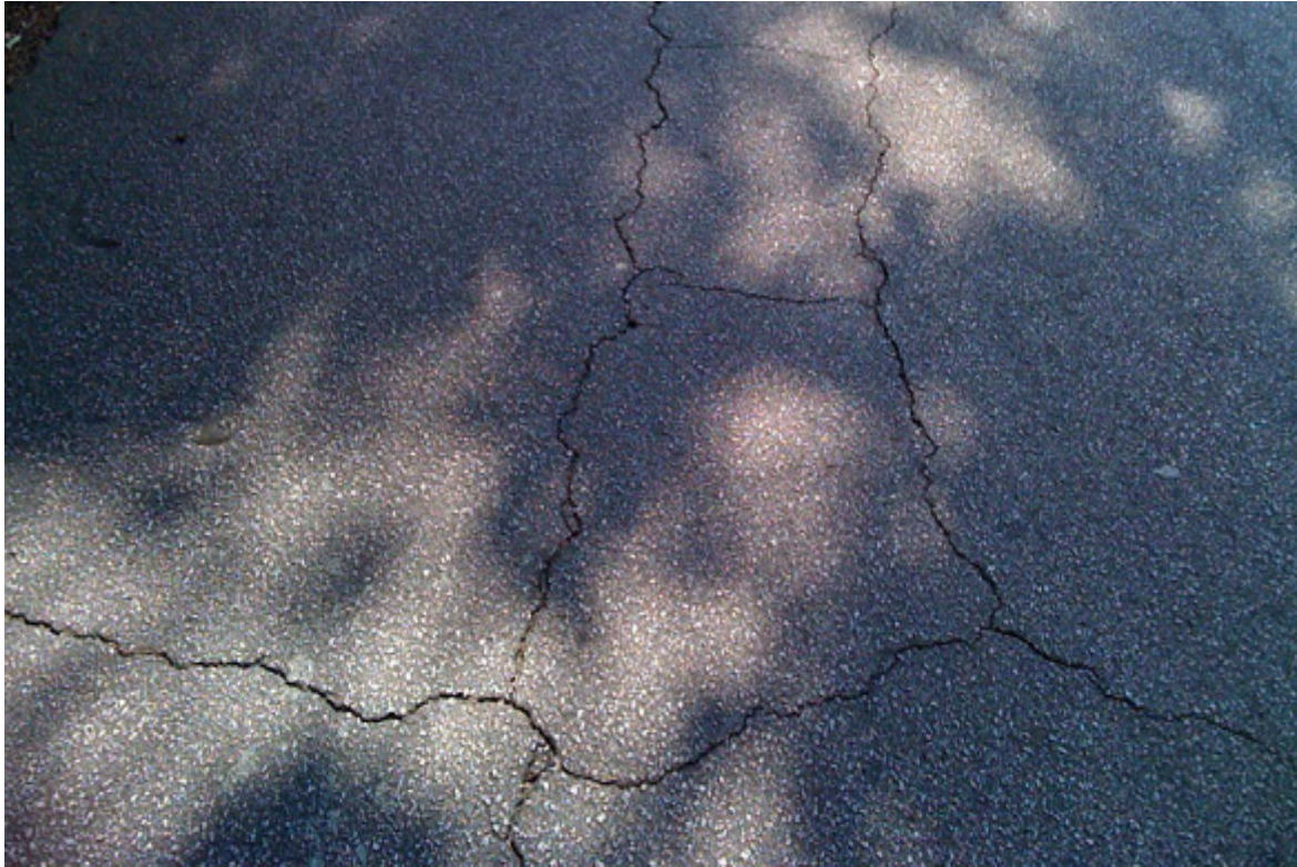
(Y) Lock Cracking
